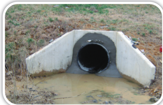
The above picture shows sliplining through a wing wall. An end seal with fill pipes is under construction.
